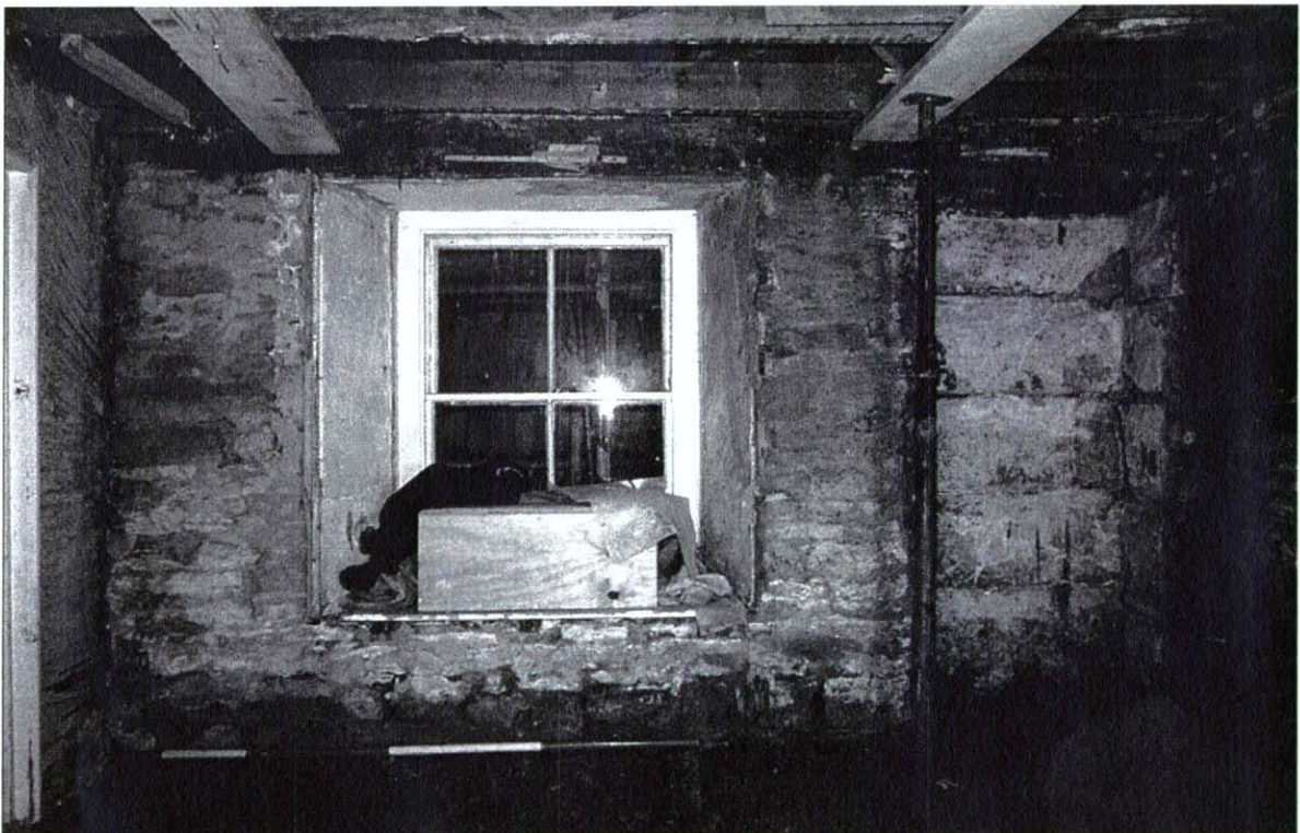
Plate 6 Ground floor LH room (N wall, altered window opening and blocked doorway).
