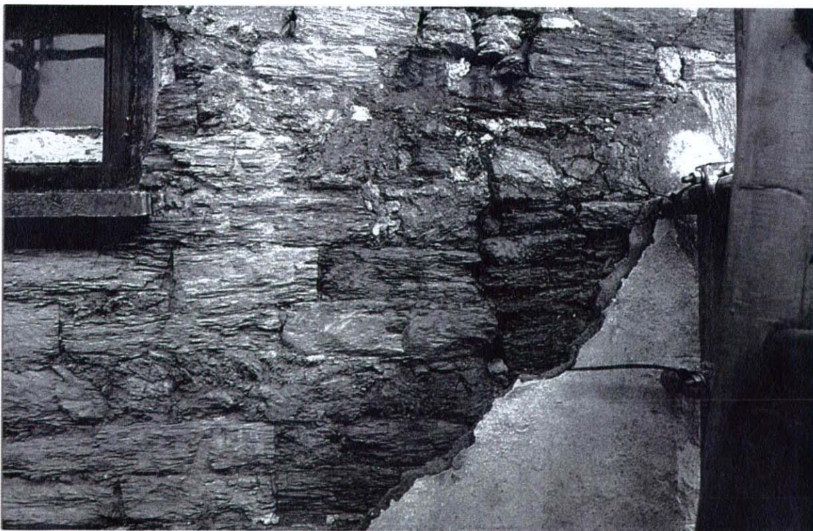
Plate 28 Front wall RH side (window alteration and evidence of rebuilding + remains of incised render).
