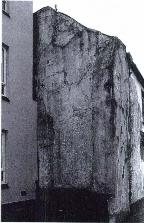
Plate 3 E gable end (pre works). Cracked and failing cement-based render obscuring structural problems of much of the wall. Gable later dismantled to eaves level.
