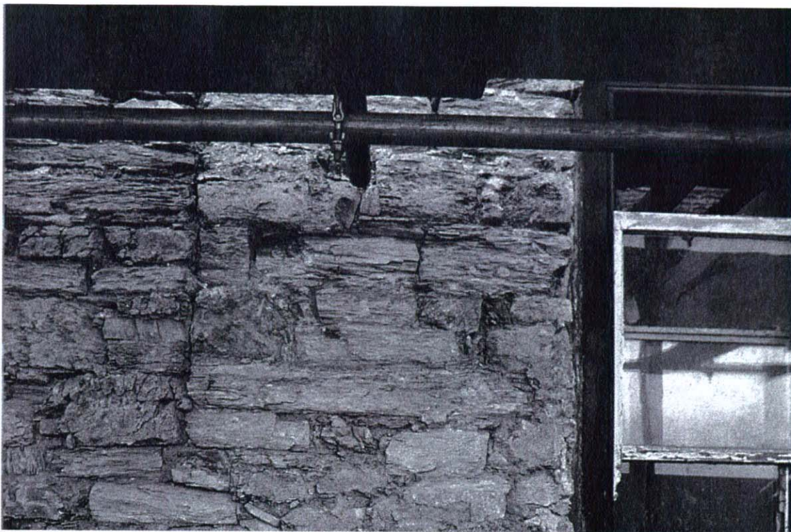
Plate 27 Front wall (1 st floor LH side showing blocked window).
